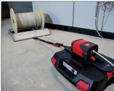
RUNPOMETER RM35 with connecting pad and belt fixed to cable drum roller PRO
